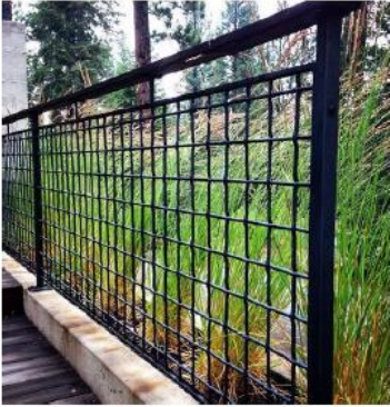
Steel & Wire Mesh Guardrail System
