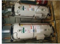
BOILER TANKS PER BLDG BLDG 'A' IN UTILITIES ROOM BLDG 'B' IN MAINT. GARAGE
