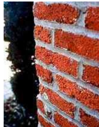
DAMAGED SANDBLASTED MASONRY
