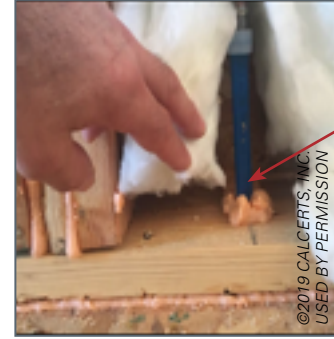
Insulation is not cut to fit behind and around obstruction to fill up cavity.
