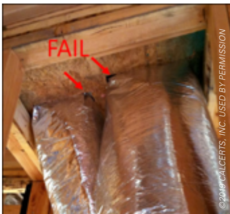
The lack of air-barrier sealing around this ductwork does not comply with QII requirements.
